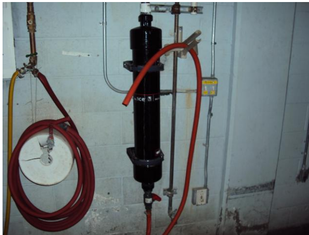
FIGURE 3. INSTALLED REALICE SYSTEM
